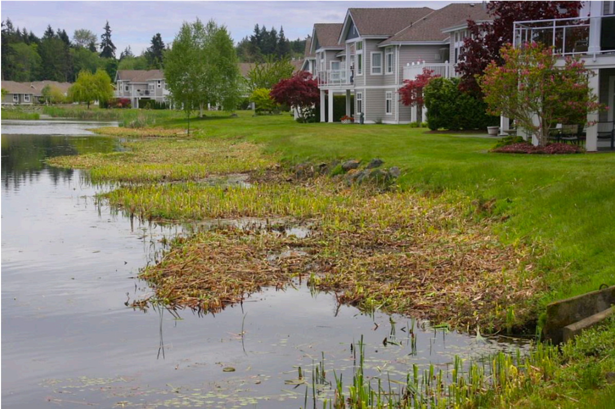
Fig. 4: One example of cattail encroachment and shoreline “creep” requiring cattail removal and later dredging-out.
