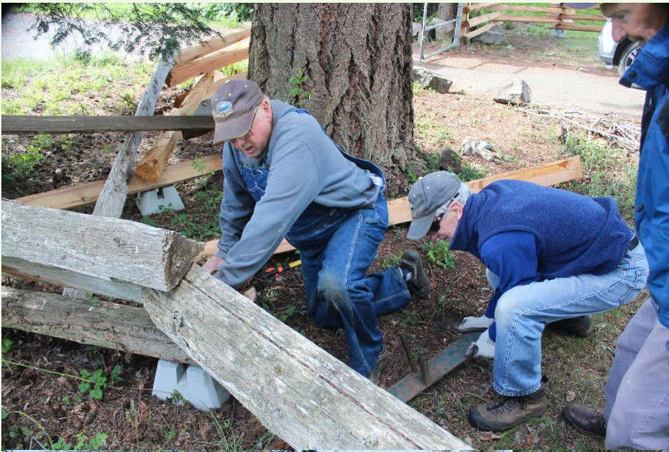
Rebuilding privacy fences and the snake rail fence at Three Bridges Pond.
